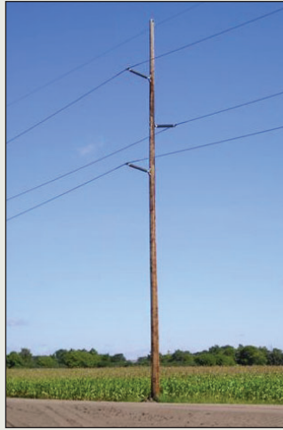
69-kV/115-kV transmission structure
