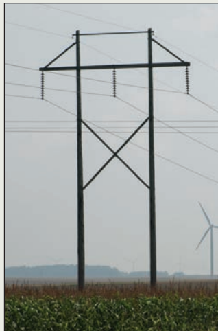
230-kV/345-kV H-frame transmission structure
